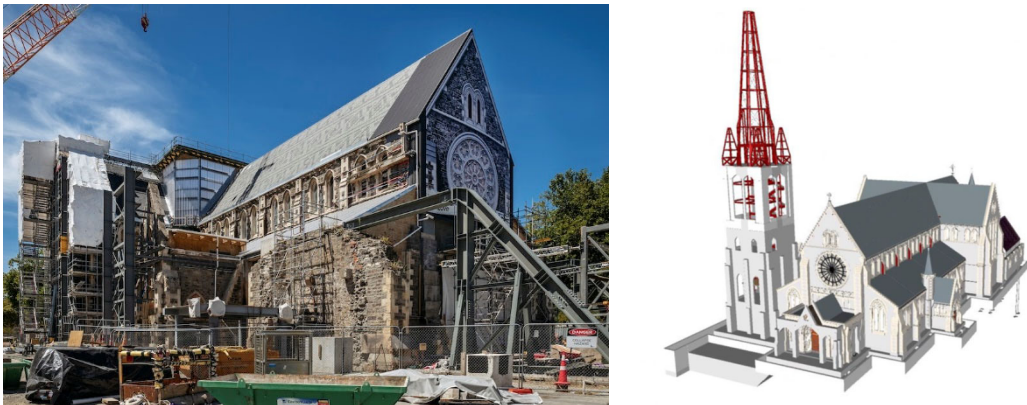
Figure 3. Earthquake repair including base-isolation of historic Christ Church Cathedral. Left: building under repair. Right: graphic of digital model used for engineering analysis.
