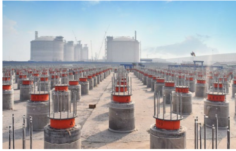
Figure 21 Seismically isolated LNG tank structure
