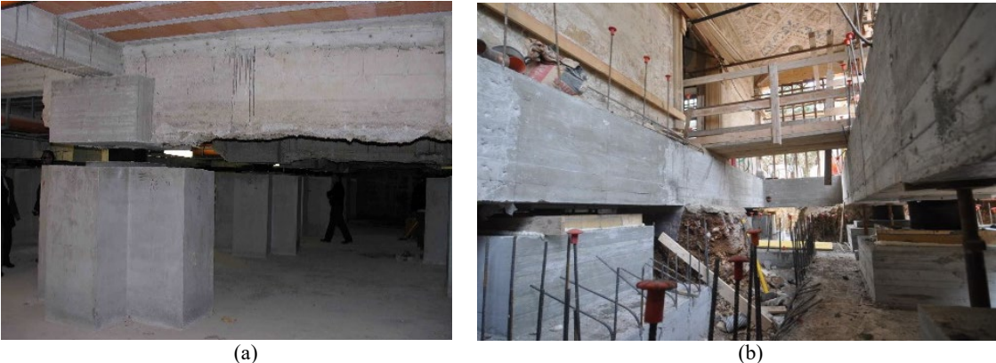
Figure 5. Seismic isolation with (a) a new sub-foundation (courtesy G. Mancinelli) and (b) two new sub-foundations (courtesy FIP Industriale and R. Vetturini).
