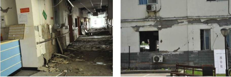
Figure 2 Two damaged non-isolated inpatient buildings in Lushan County Hospital
